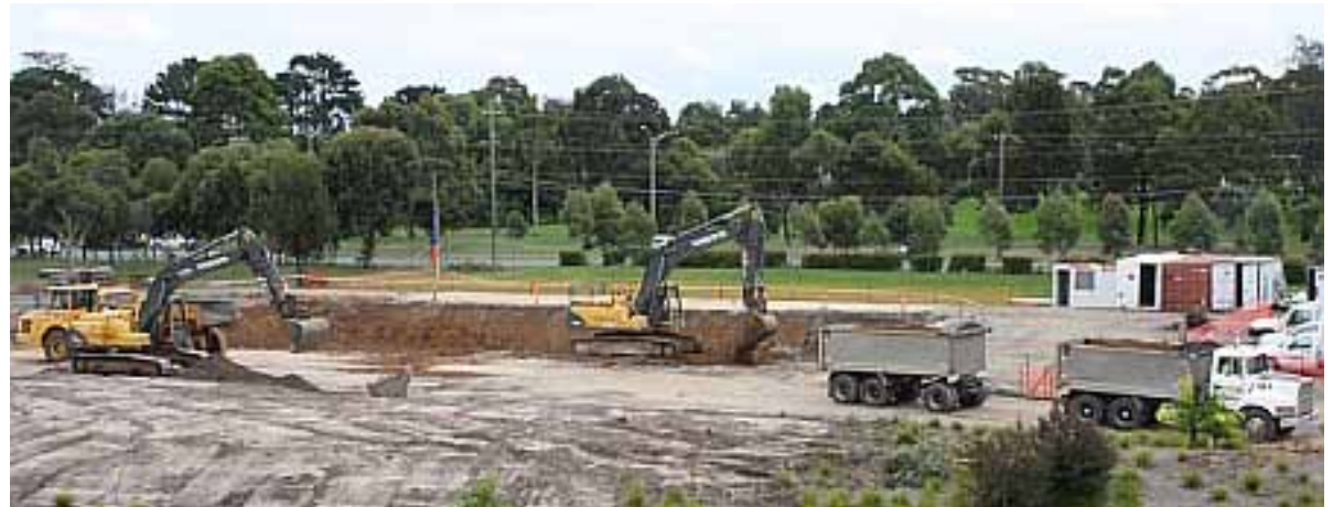
[18 January 2011]: views of the excavation work in the gravel carpark near the synchrotron entrance gate on Blackburn Road.
