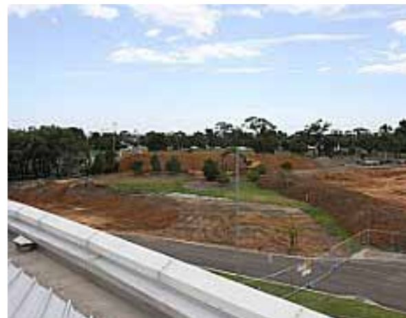
[1 February 2011] L to R: excavation works for road relocation and NCCS building.
