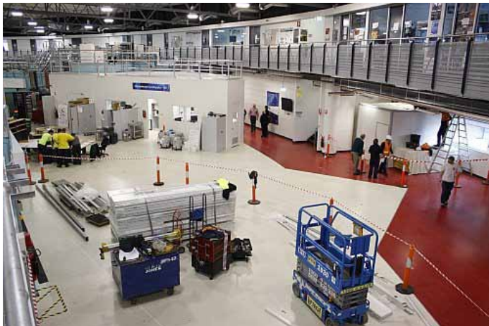
Preparing for construction (looking counterclockwise from the XFM beamline roof towards the MX user cabins)
