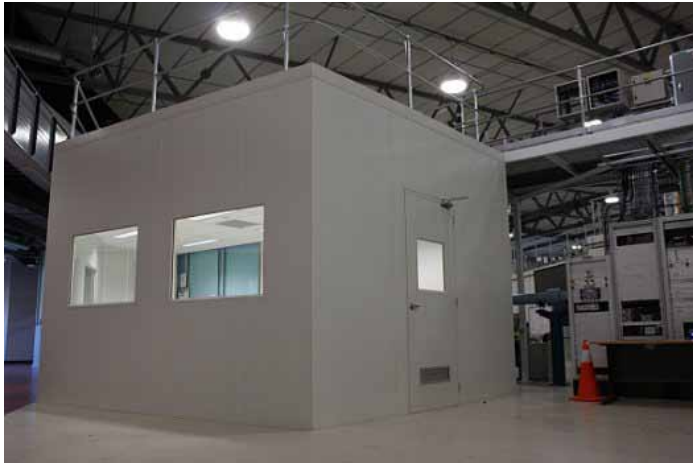
Worm's eye view of the main user cabin under construction (looking clockwise from the MX beamlines).
