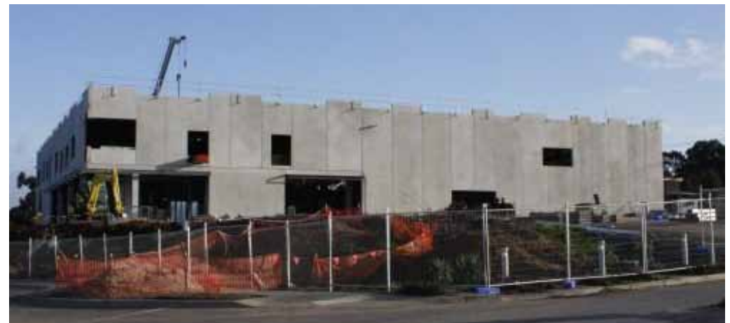
[12 August 2011]: the north wall of the NCSS building.
