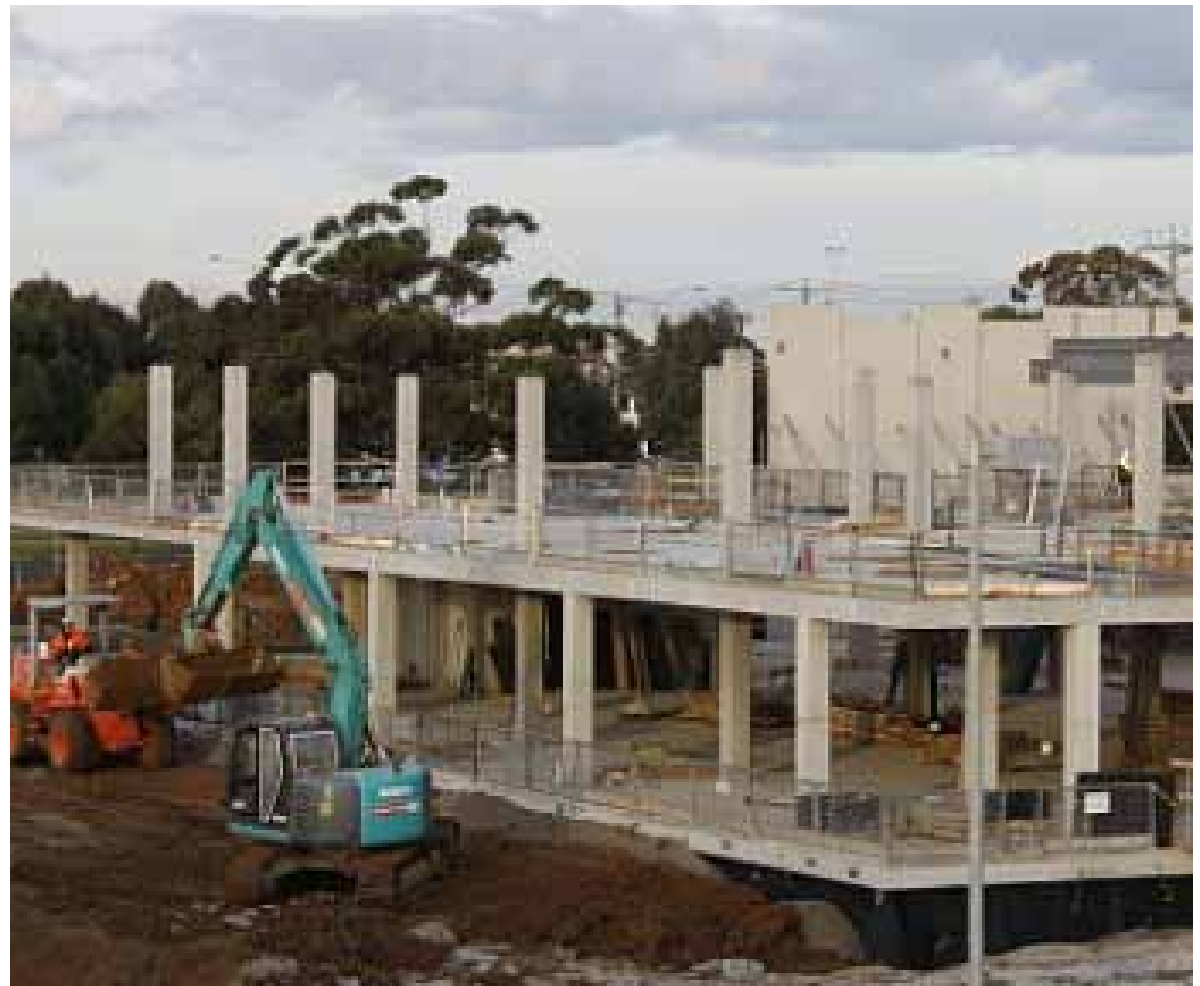
(1 July 2011): using dirt stockpiled from the excavation to fill in the trench around the NCSS building.
