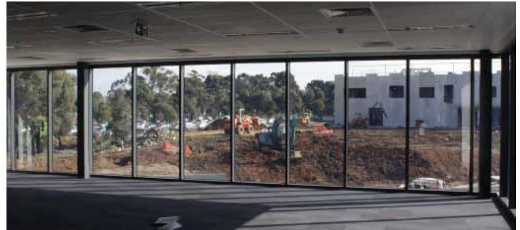
[11 August 2011]: NCSS building viewed from the first floor of the technical support laboratories building.
